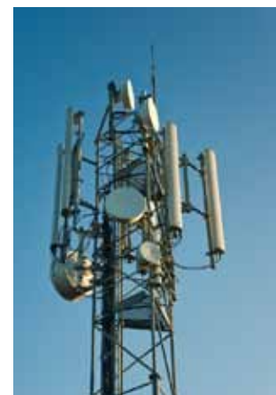
(2) BTS: Base Transceiver Station (relay emitters)
